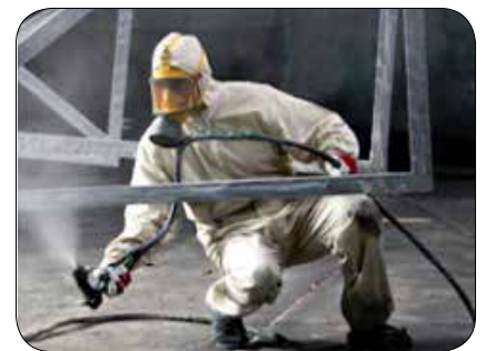
Dedicated Paint Booth
